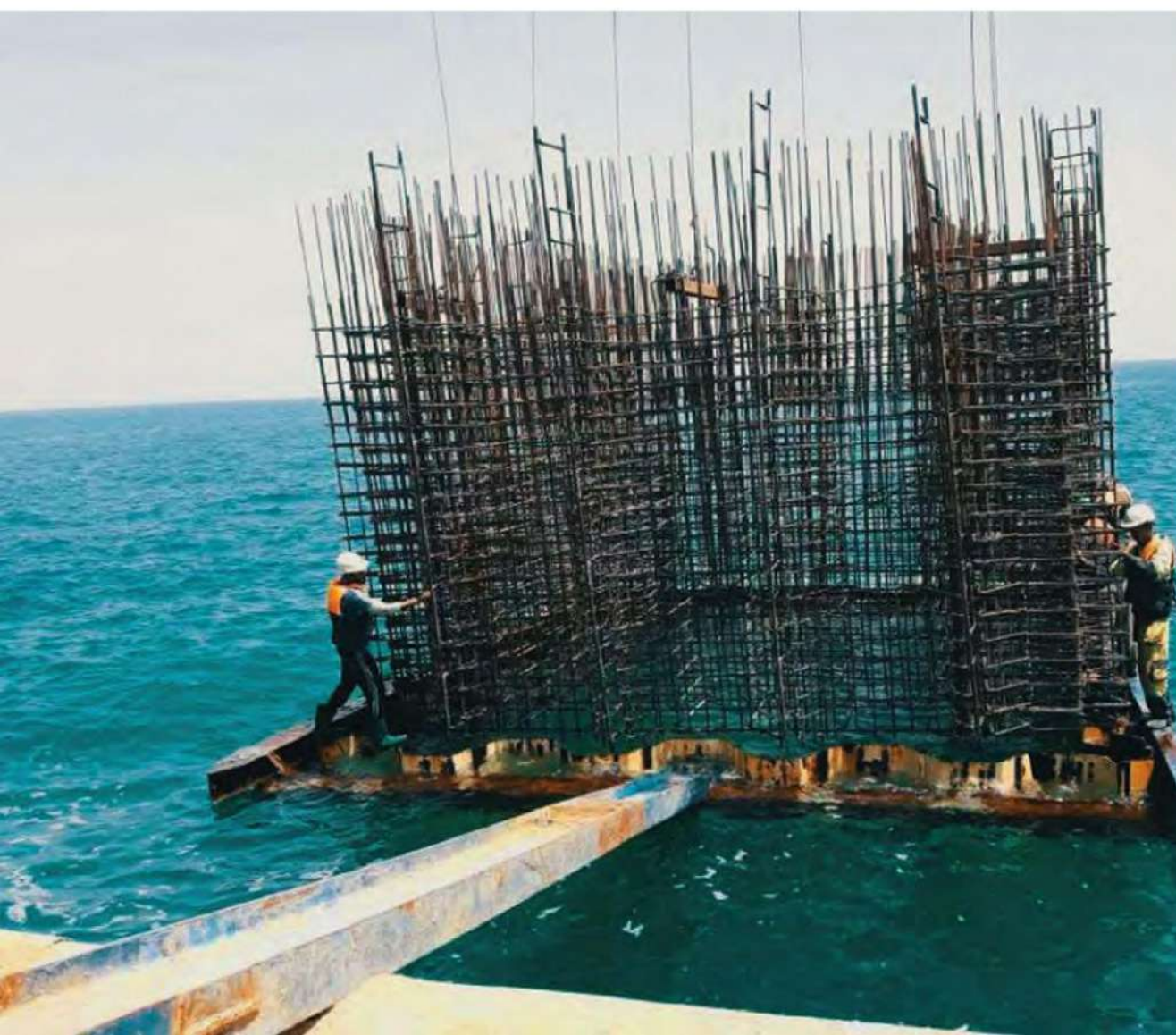
Development of EHC - OPC gas tankers berth Location: Elsokhna, Gulf of Suez, Egypt Client: OPC - EHC
